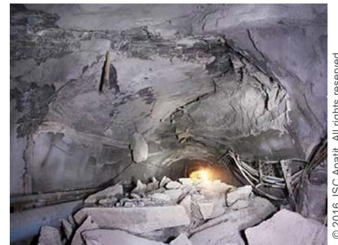
Example of a rockburst event aftermath in a drift.
